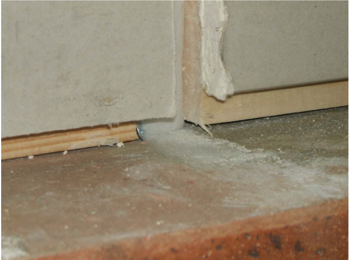
Photograph 2: Partially Unsealed Partition Close-Up
