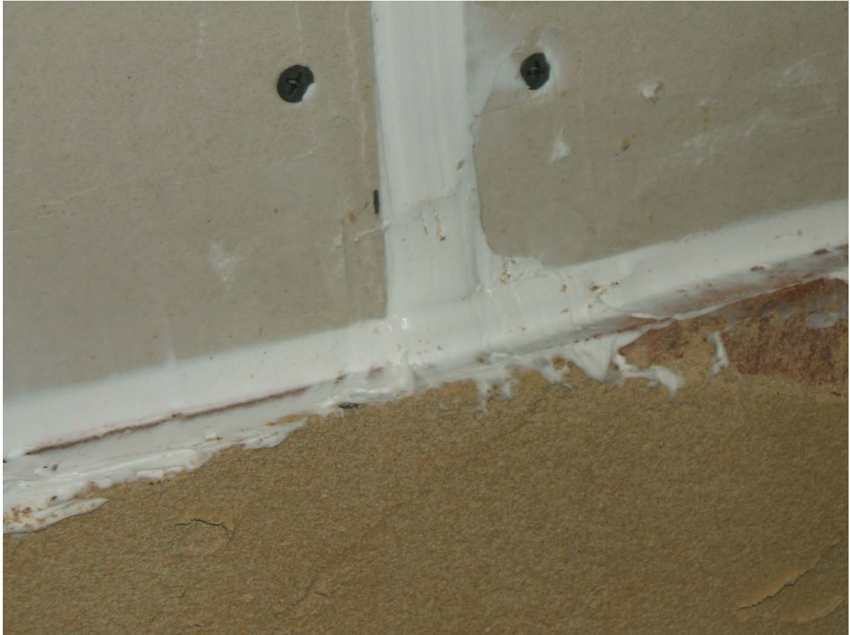
Photograph 3: Partition Sealed Close-Up
