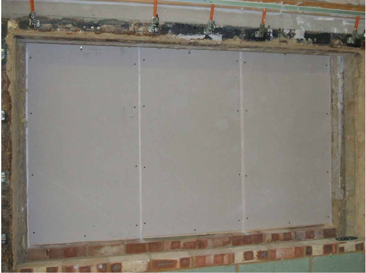
Photograph 1: Partially Unsealed Partition
